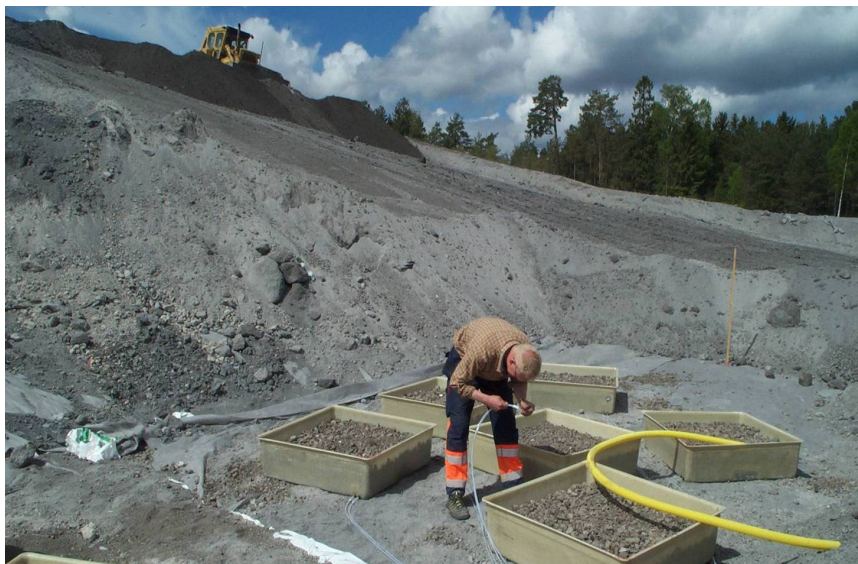
Figure 3 Lysimeter boxes with hoses and protection hoses installed below the liner of fly ash.
